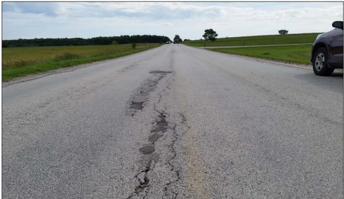
Center line longitudinal and driving lane longitudinal cracking
