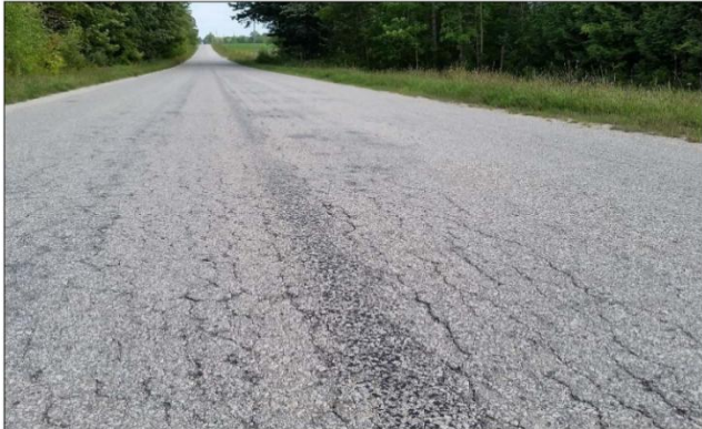
Alligator cracking throughout road
