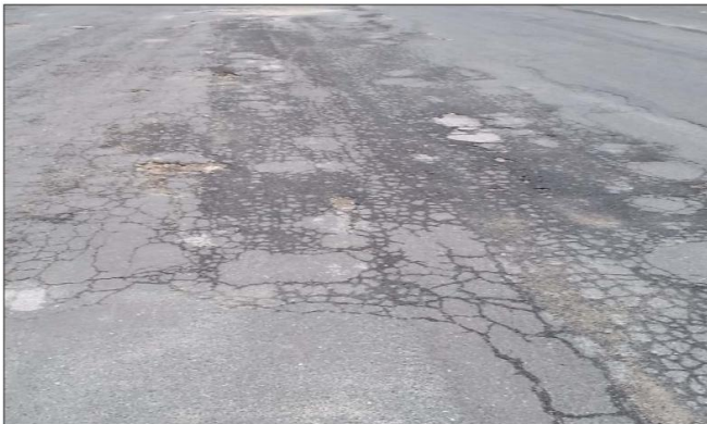
Cover aggregate loss through pavement indicating poor base
