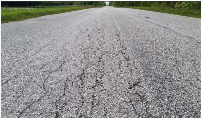
Alligator and map cracking
